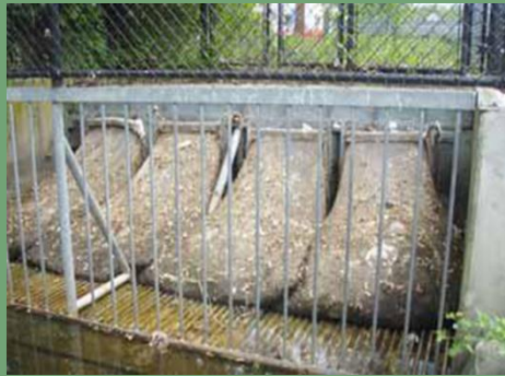
Multiple net filters capture organic matter at the end of a storm drain system
