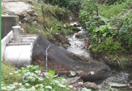
Bag filter installed at outfall in the Town of Easton
