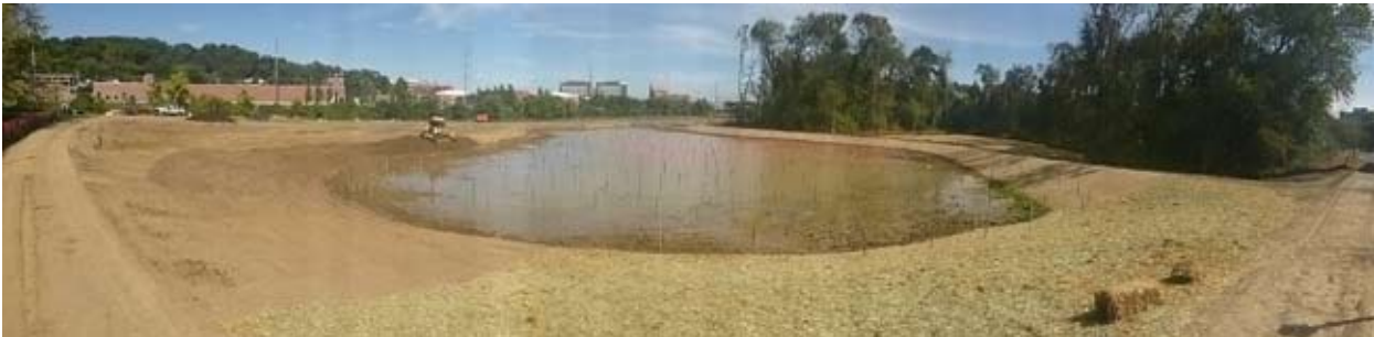
Four Mile Run Wetlands Restoration project in progress. At this stage, the wetlands have been restored and the plantings were being put in.
